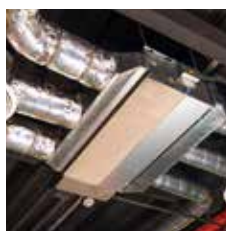
Air renewal units
